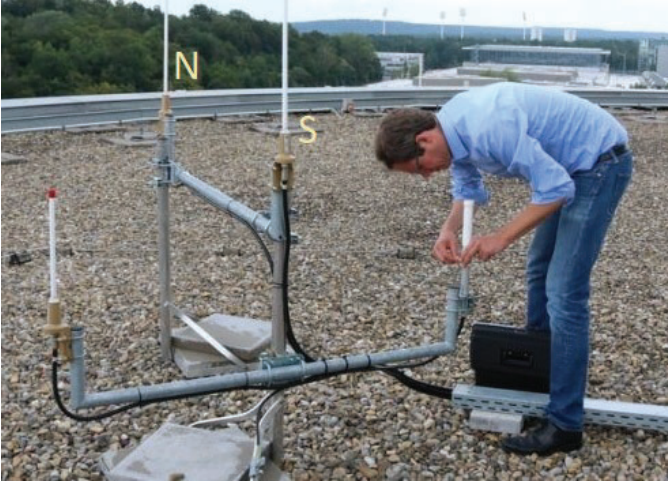
Fig. 6. Receiver 21 on the rooftop of the tallest fair building. The Cloud RAN antennas are the two antennas in the center of the picture. The spacing between the antennas is exactly four wavelengths, i.e. 1.38 m with N/S.
